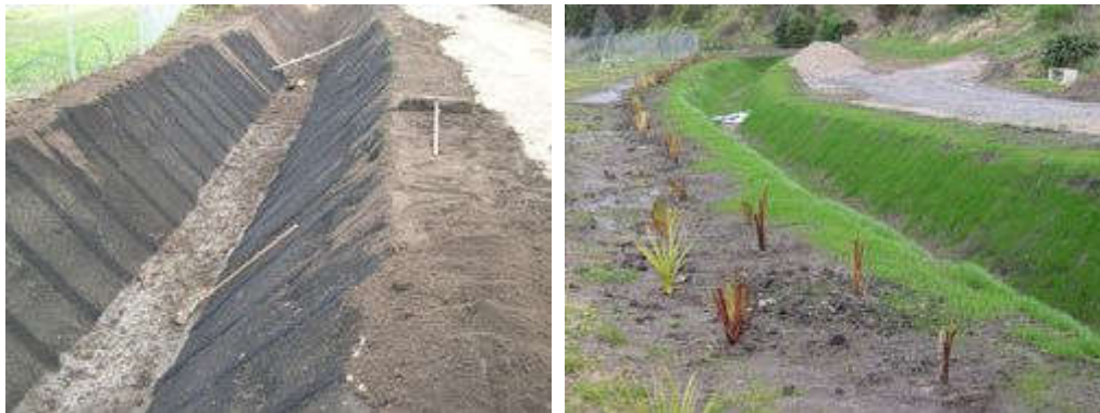
Photo: mats that have been laid on a slope to prevent soil erosion, finished result
